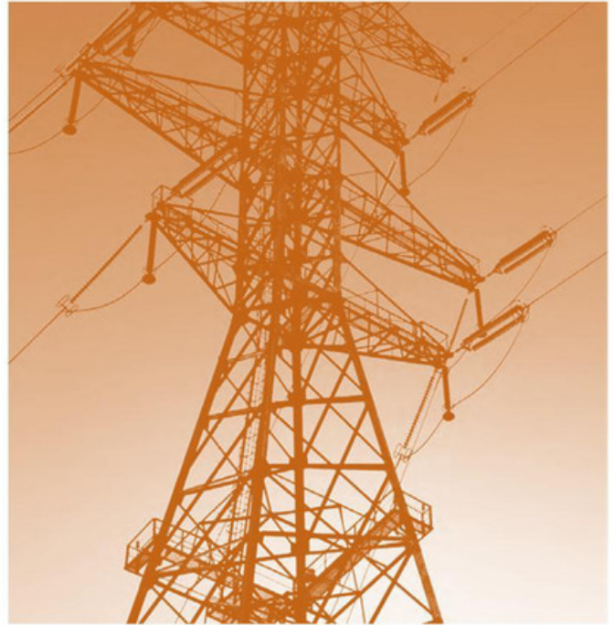
KCP&L and GMO's electric utility system has approximately 3,600 circuit miles of transmission lines
