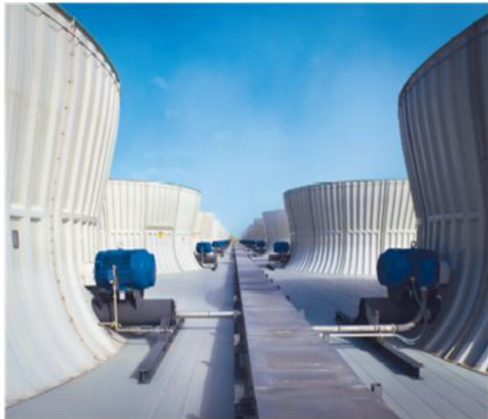
Iatan 2 cooling tower fans. The use of a cooling tower for condenser cooling is an integral part of Iatan's environmentally friendly zero liquid discharge operation.
